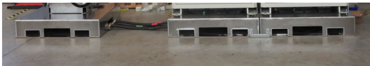
Figure 2. Representative example of an in-laboratory EVSE installation.
