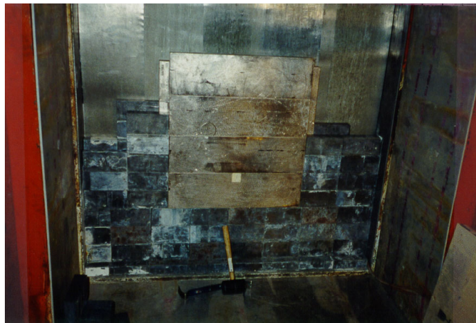
Figure 10. Cadmium thermal neutron shield and bismuth-lead gamma shield during installation at WSU.
