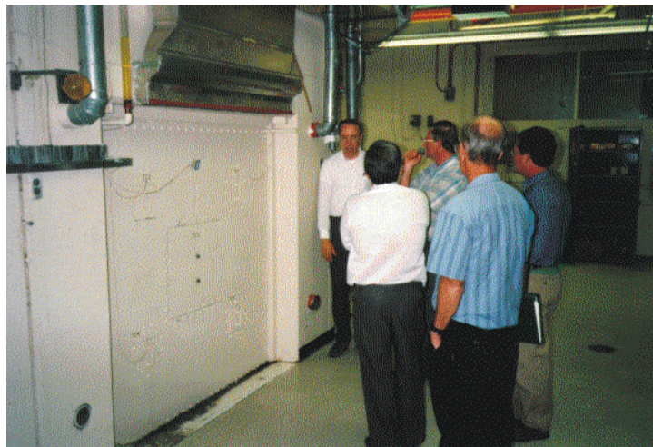
Figure 2. Final thermal column shield and adjacent floor area at the WSU TRIGA facility prior to modifications.
