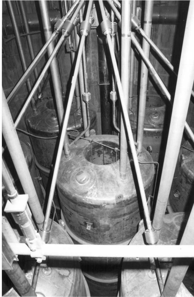
Figure A-7. Distribution piping for Calcine Solids Storage Facility VI (84-680-1-6).
