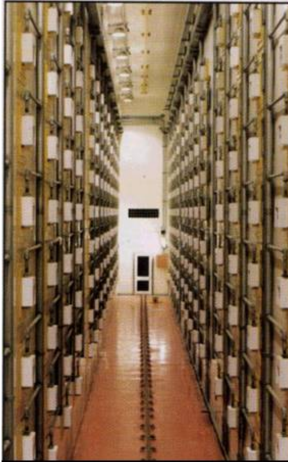
Figure B-1. Remotely operated store for Pure PuO 2 in welded stainless steel canisters at BNFL Sellafield.
