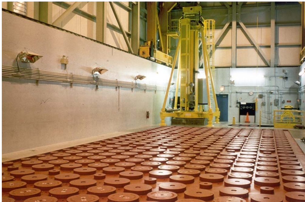
Figure A-5. Fort St. Vrain modular vault dry store (MVDS) showing charge face.
