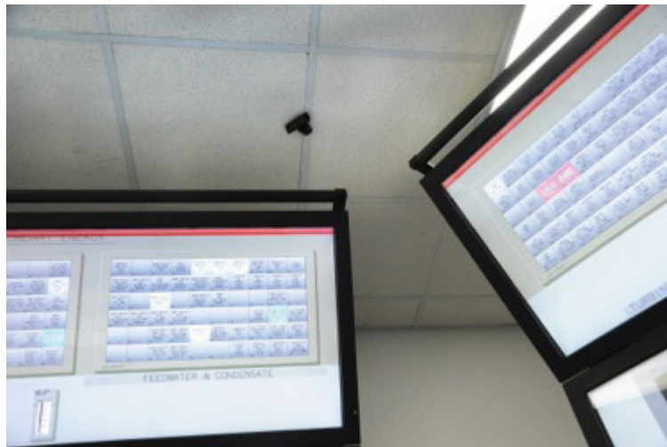
Figure 8. Placement of a Ceiling Camera for Observation.
