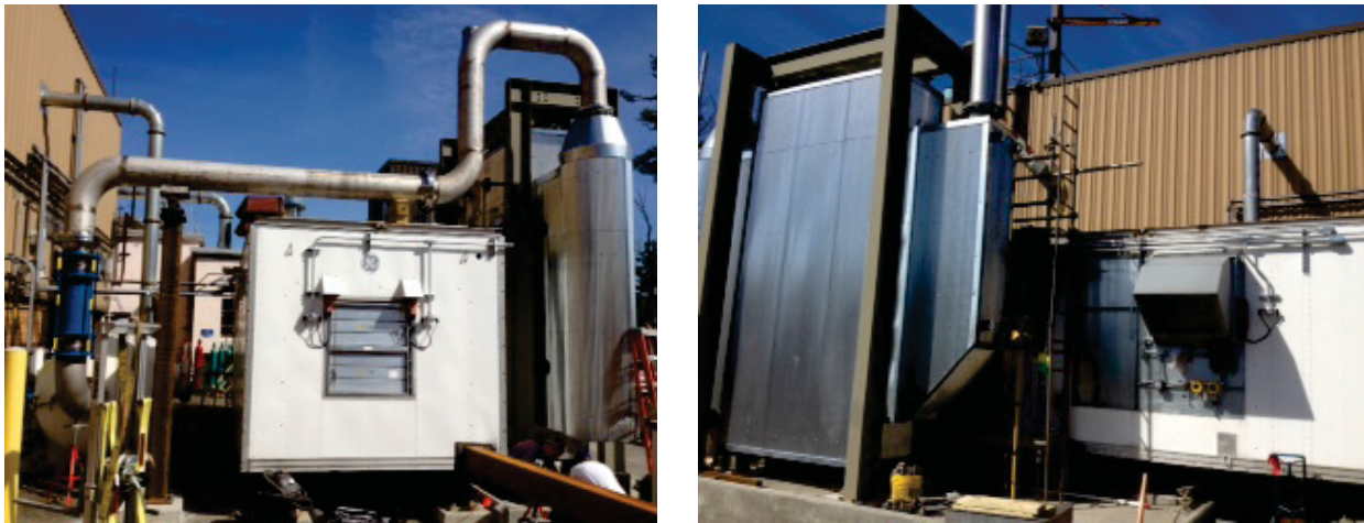
Figure 24. Direct evaporator installed at GE test facility.
