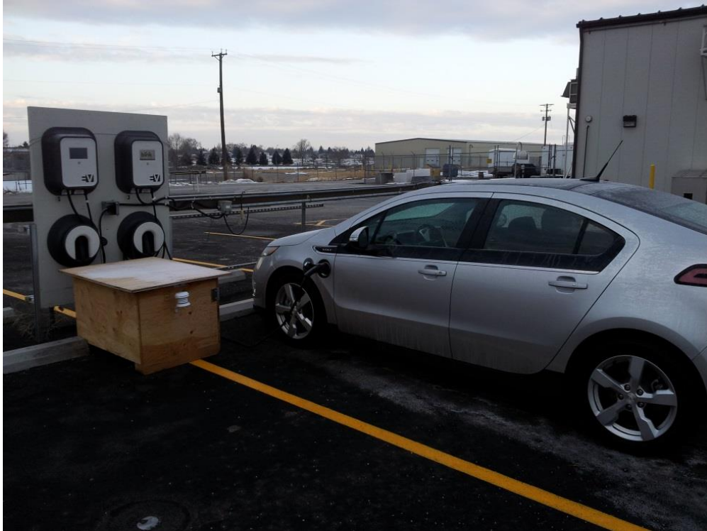
Figure 2. Volt charging location with charging equipment in weather-proof container.
