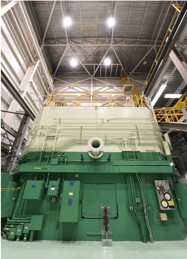
Transient Test Reactor
