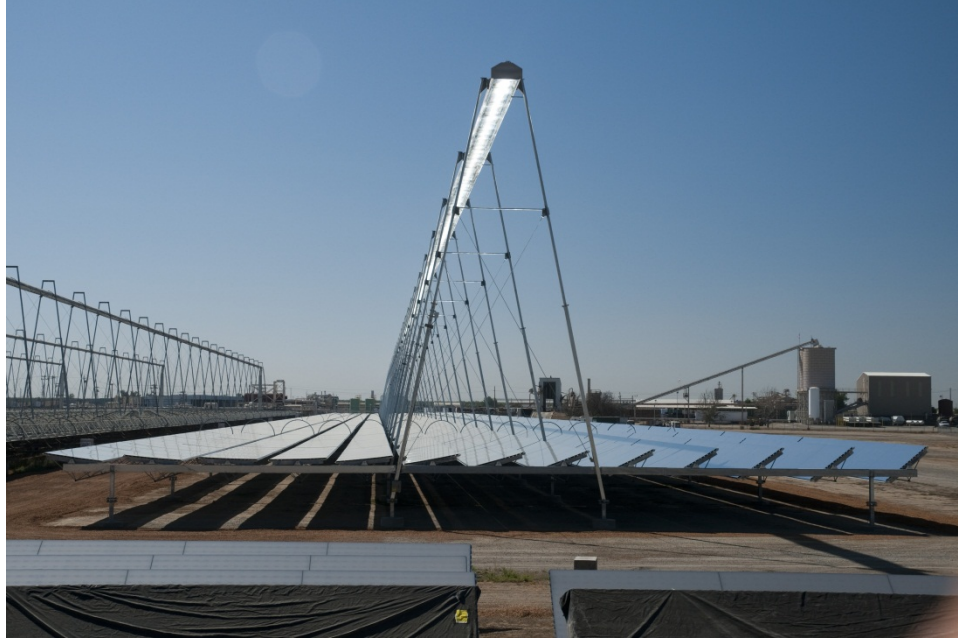
Figure 7. Linear Fresnel system showing ground-mounted flat mirrors and a fixed overhead receiver (Areva Solar, NREL PIX 19883).
