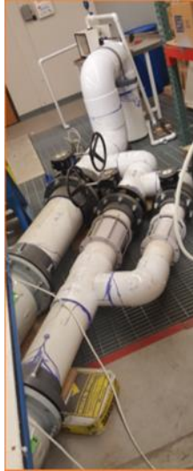
Figure 5-13 ISU Flood Testing Facility Pump System 1 - 3-Channel Path at the Outlet [34]
