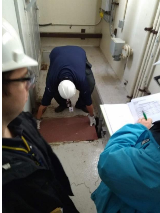
Figure 5-4 Access to the Cable Tunnel in the EDG Room (Courtesy of Oyster Creek NPP)
