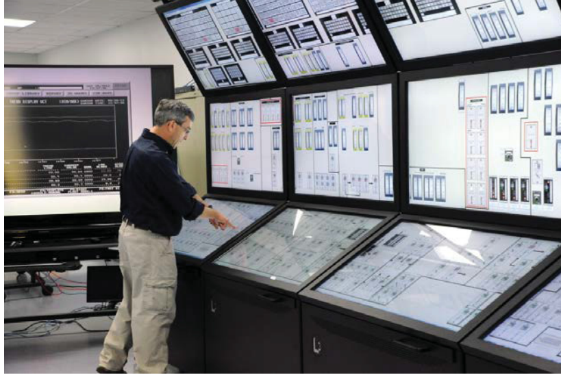
Figure 5. HSSL used to evaluate digital upgrades in a hybrid control room
