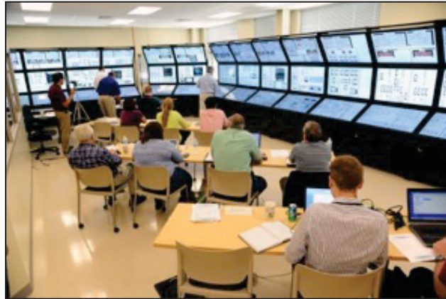
Figure 6. HSSL used for an operator work shop.
