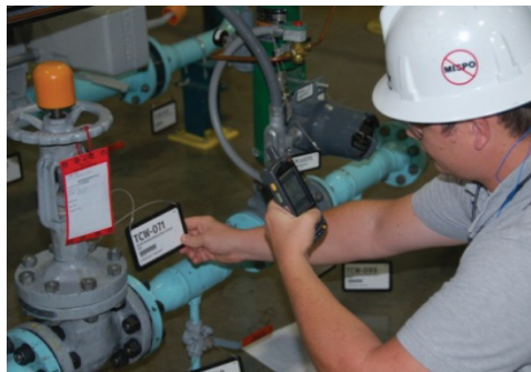
Figure 8. Operator at Catawba Nuclear Station using hand-held technology for component identification.
