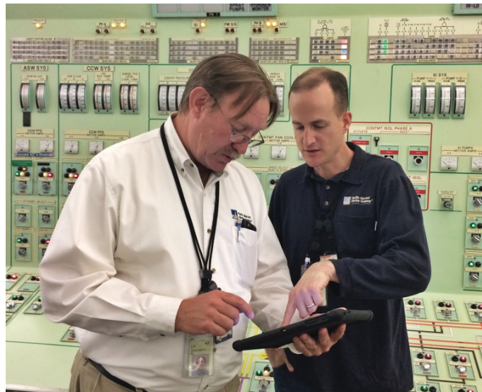
Figure 10. A control room operator and a field operator at Diablo Canyon Power Plant discuss a procedure using the computer-based procedure system on the hand-held device.
