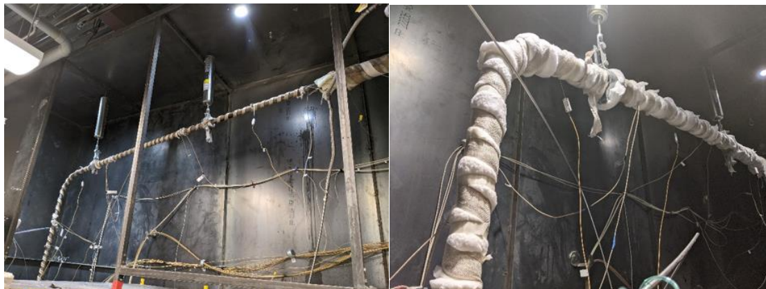
Figure 4. New heat tape on the loop and new insulation.
