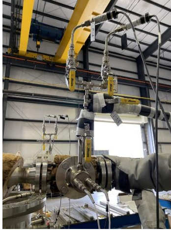
Figure 19. Pressure and RTD manifolds located on the inlet and outlet (siphon and vent) of the drying chamber.
