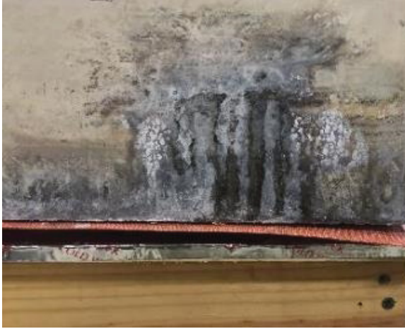
Figure 5. Damage location 1—cracking and powder effluence.
