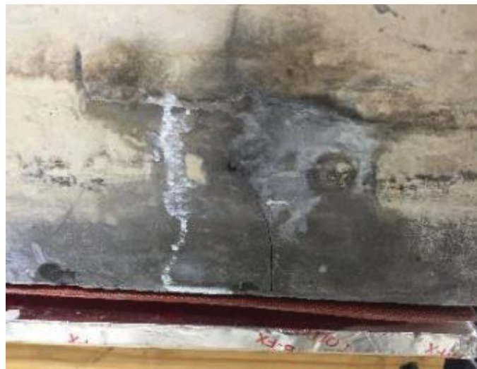
Figure 7. Damage location 3—cracking and powder effluence.
