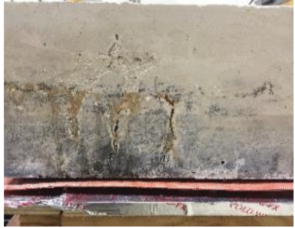
Figure 6. Damage location 2—clear gel effluence.
