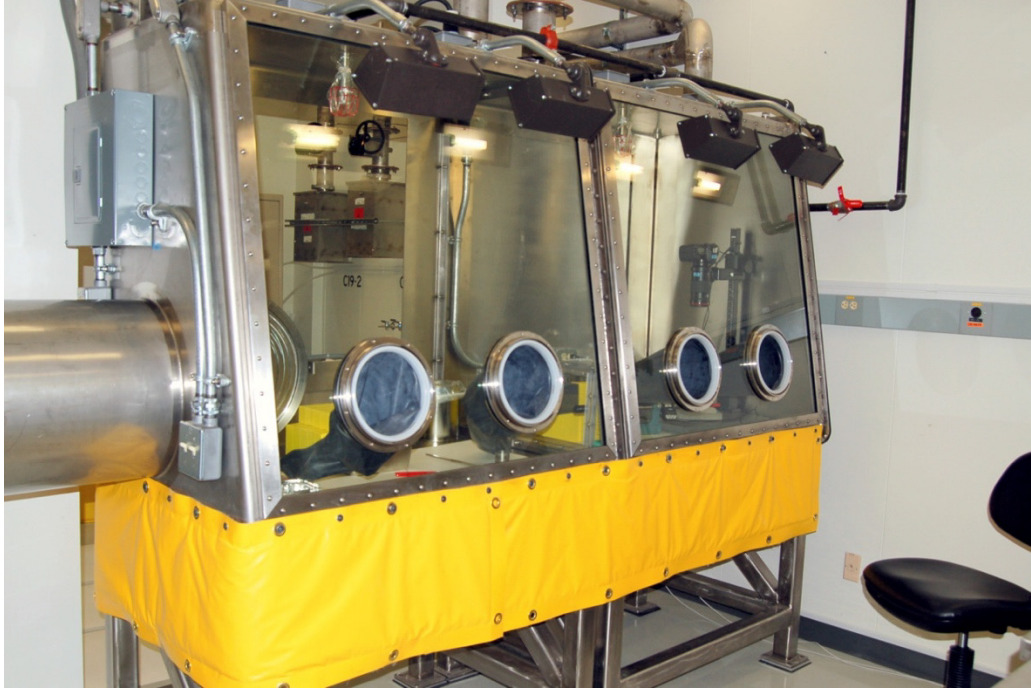
Figure 1. CCL glovebox used to visually inspect graphite samples, perform initial dimensional measurement, and repackage samples for storage in the irradiated graphite vault located in Lab C-19
