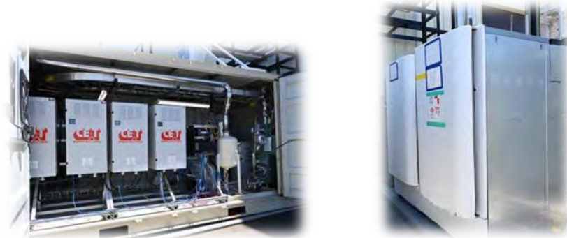
Modular Systems / Balance of Plant
